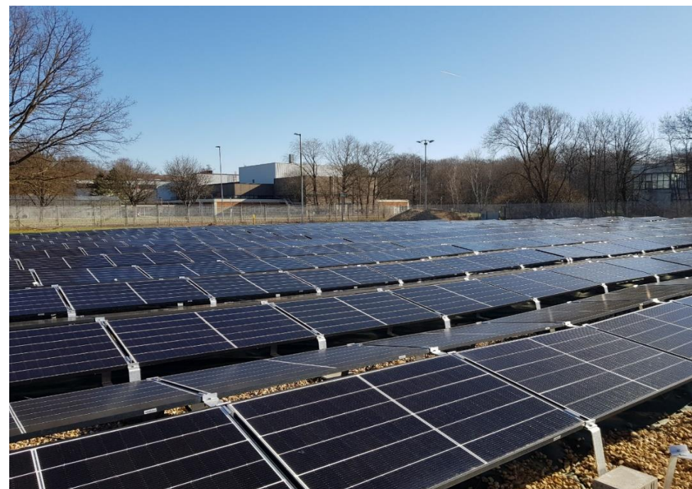
PV FIELD Sunny Tripower CORE2 1.1 MWp
