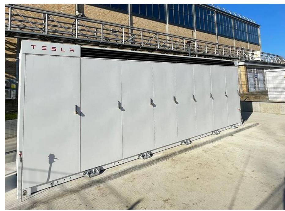
High-energy battery Tesla "Megapack" 500 kW / 2.5 MWh
